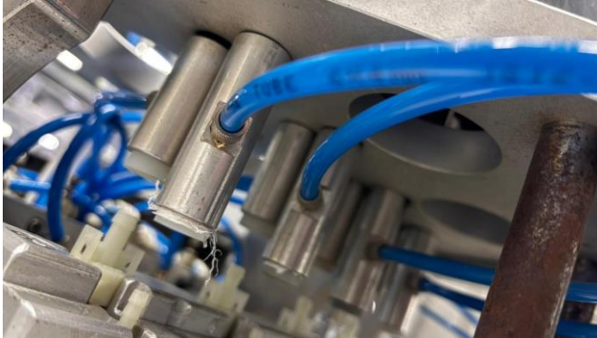
Figure 4 Pressure Verification Setup for Safety Valve Inspection
