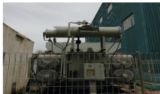
Gambar 2. Generator Transformator Unit 1 PLTU Tanjung Balai Karimun
