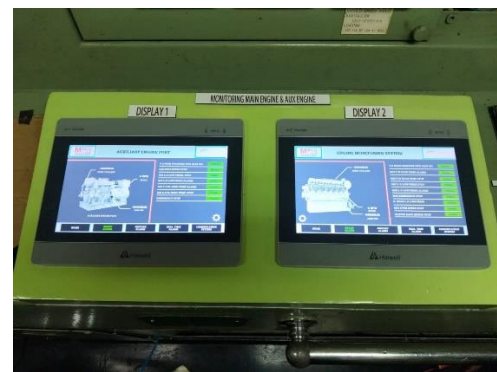
Figure 8. Actual Alarm monitoring system Cloud SCADA
