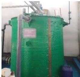
Gambar 3. 3 Reverse Osmosis (RO) Cleaning Tank
