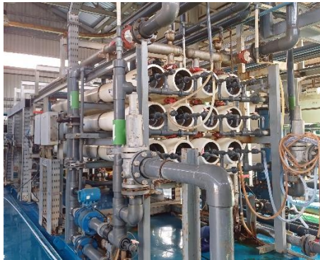
Gambar 2. 1 Membrane Sea Water Reverse Osmosis (SWRO)
