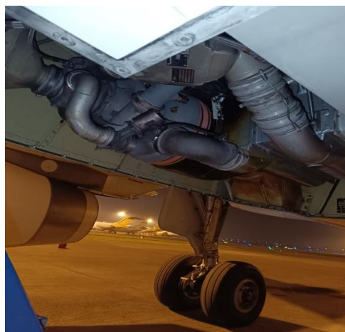
Gambar 1.2 Air Conditioning Pack 1 Bay
