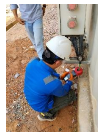
Figure 12. Final Commissioning and Testing, Workshop 3 & 4, PT VME Process
