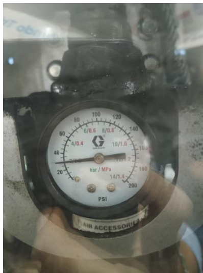
Gambar 5 Setting Pressure pump
