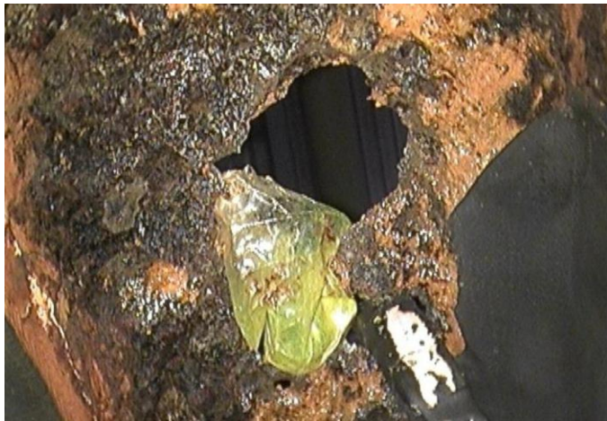
Gambar 4. Kebocoran Water Box Kondensor PLTGU Tj. Uncang
