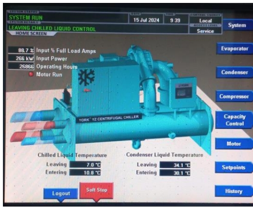
Figure. 1. Chiller Machine Screen Display
