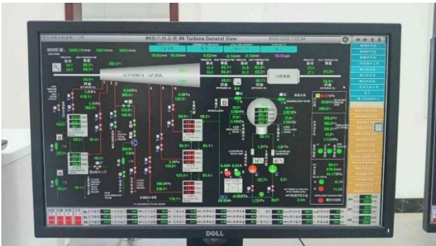
Gambar 9. Distributed Control System (DCS) Unit 4 PT BAI (Dokumentasi Pribadi)
