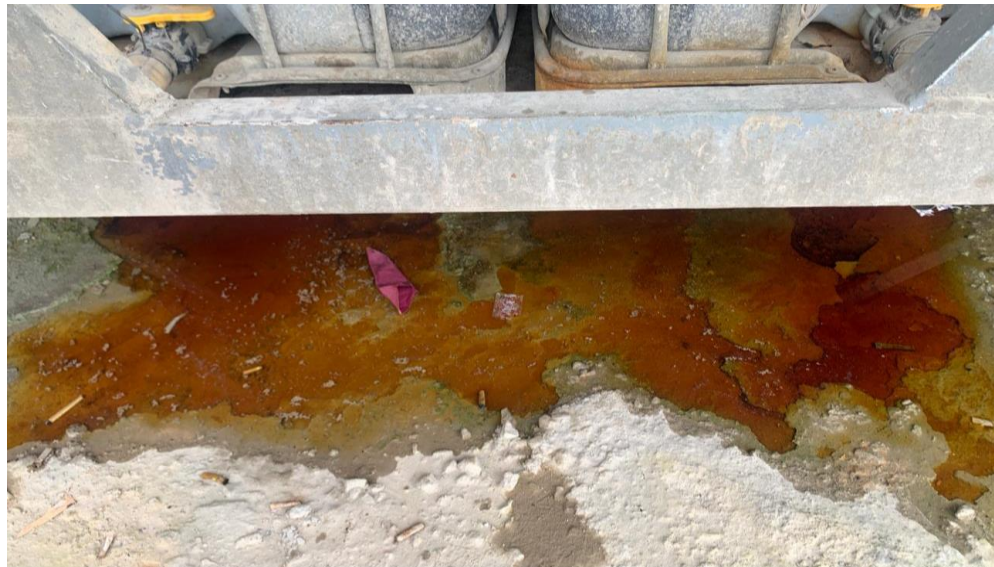
Gambar 7 Admix tumpah di lantai batching plant
