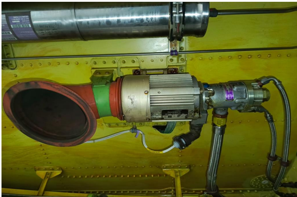
Gambar 3. Standby Electric Motor Driven Pump
