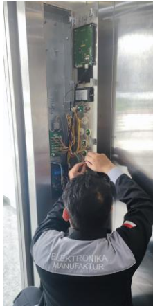
Figure 16. Installation Process of the RFID-Based Elevator Authorization System
