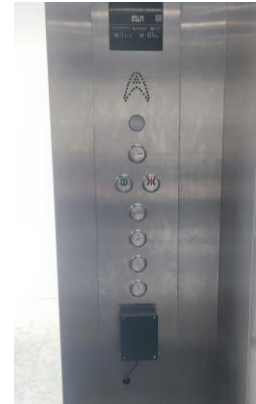
Figure 18. RFID Reader Installed on the Elevator Car Operating Panel (COP)
