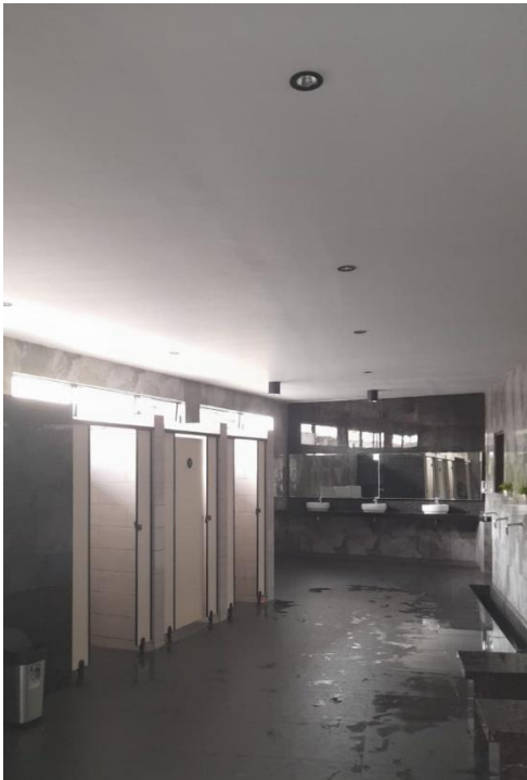
Figure 4. Mosque toilet lights
