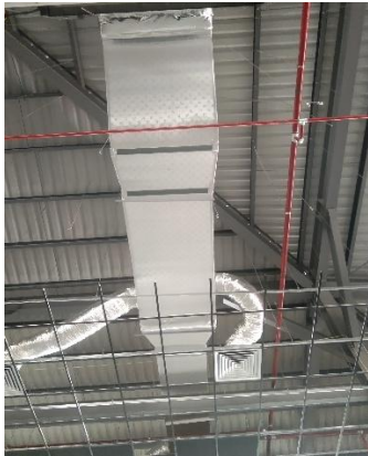
Fig. 7. The main cold air duct is insulated rectangular galvanized zinc that runs under the steel roof frame.
