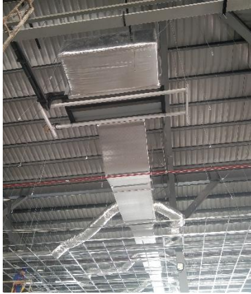
Fig. 6. Indoor Fan Coil (FCU) unit with insulated air divider (plenum) box.
