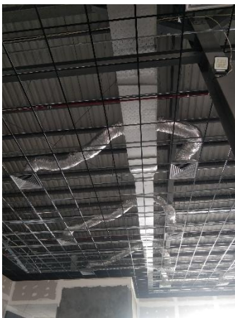
Fig. 8. Flexible branch ducts that supply air to the square ceiling vents inside the open ceiling structure.
