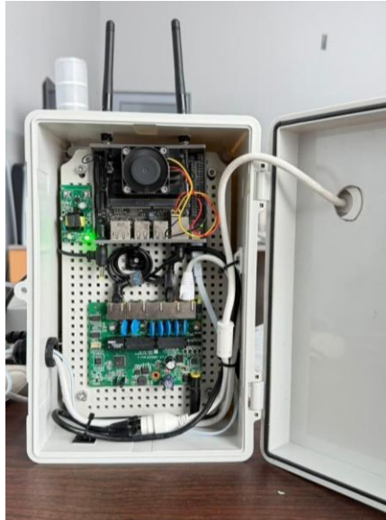
Gambar 4.4 Instalasi embedded PC
