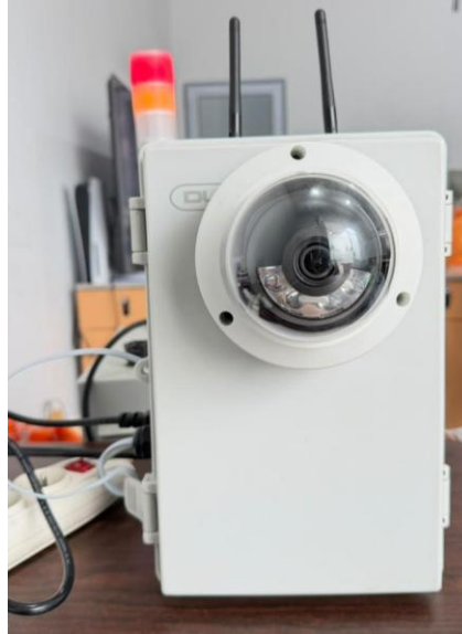
Gambar 4.5 Instalasi Surveillance Camera
