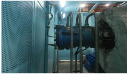
Gambar 2.8 Turbine Stop Valve
