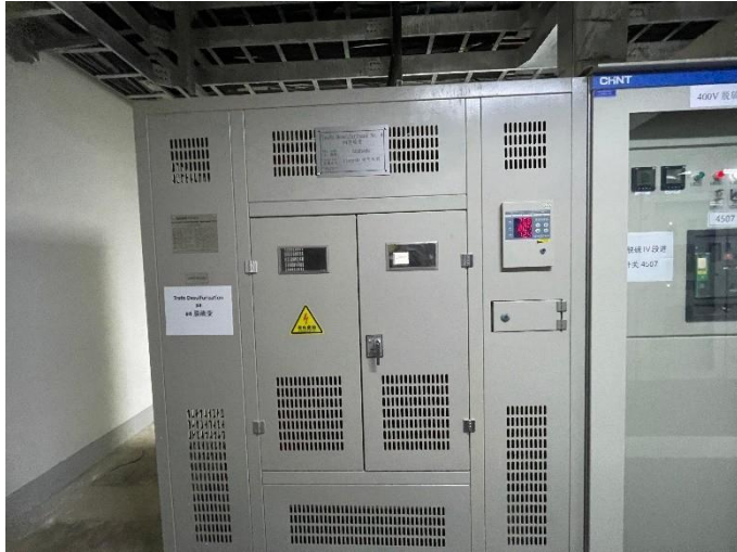
Gambar 1. Trafo Kering Desulfurization PLTU PT. Bintang Alumina Indonesia
