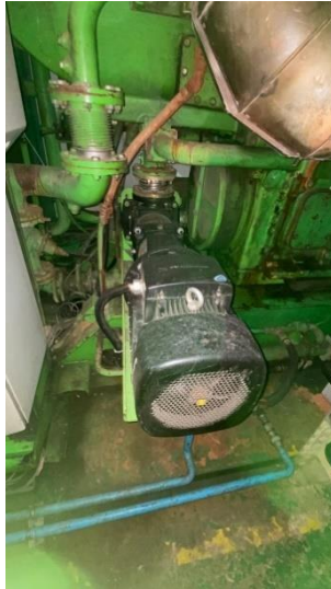
Gambar 5. Pompa Sirkulasi Air Pendingin (Jacket Water Pump)
