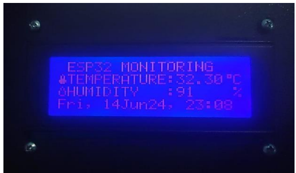
Fig 19. Temperature and Humidity Out of Limit Display
