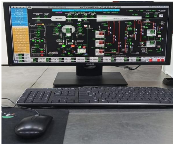
Gambar 15. Distributed Control System ( DCS )
