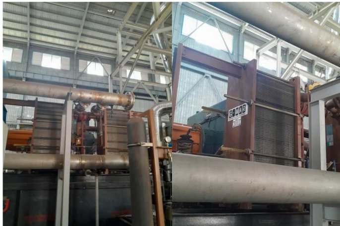
Gambar 19. Plate Heat Exchanger (PHE) di Steam Turbine Generator (STG) (sumber : Foto Pribadi)
