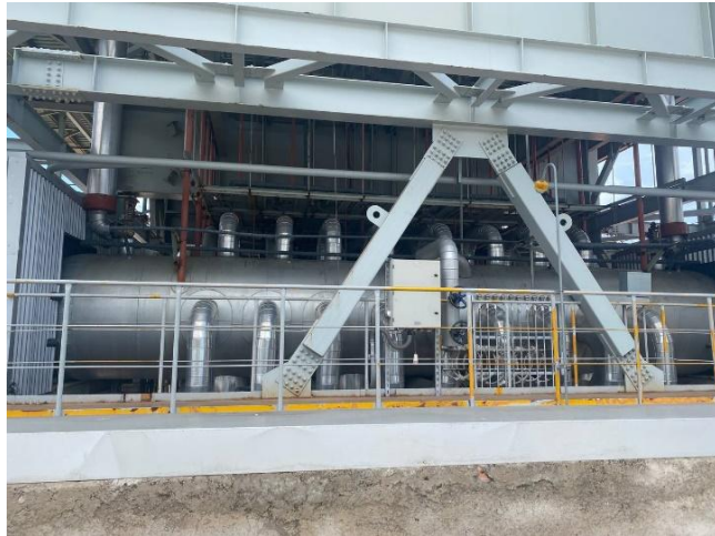
Gambar 3. Steam Drum di PLTU PT. Bintang Alumina Indonesia
