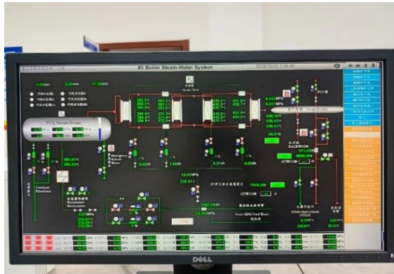
Gambar 7. Posisi Superheater di Distributed Control System
