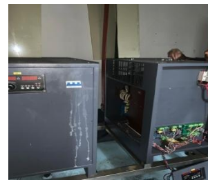
Figure 1 Improved rectifier 12volt 1200A.
