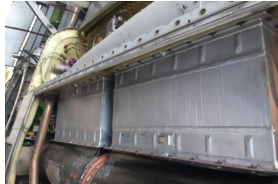
Gambar 8. lokasi heat exchanger
