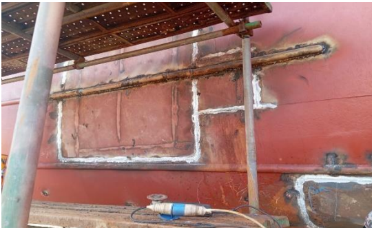
Gambar 4. Proses liquid penetrant test
