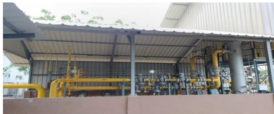
Gambar 3. Metering Regulating Station (MRS) PLTMG MCB
