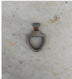
Gambar 6. Clamp Grounding Cable BCC
