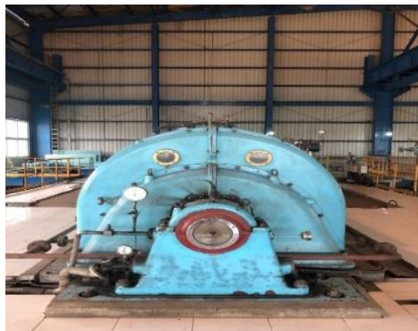
Gambar 1. Generator EOB3 Zug Ecogreen Oleochemicals
